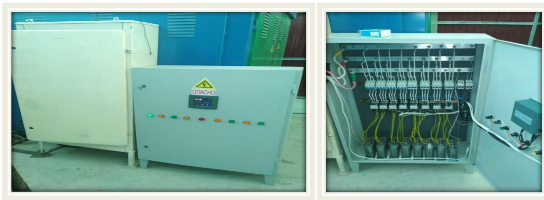
Figure 5: General view of installed capacitors for reactive power compensation in the forage grinding shop, conclusion and discussion
