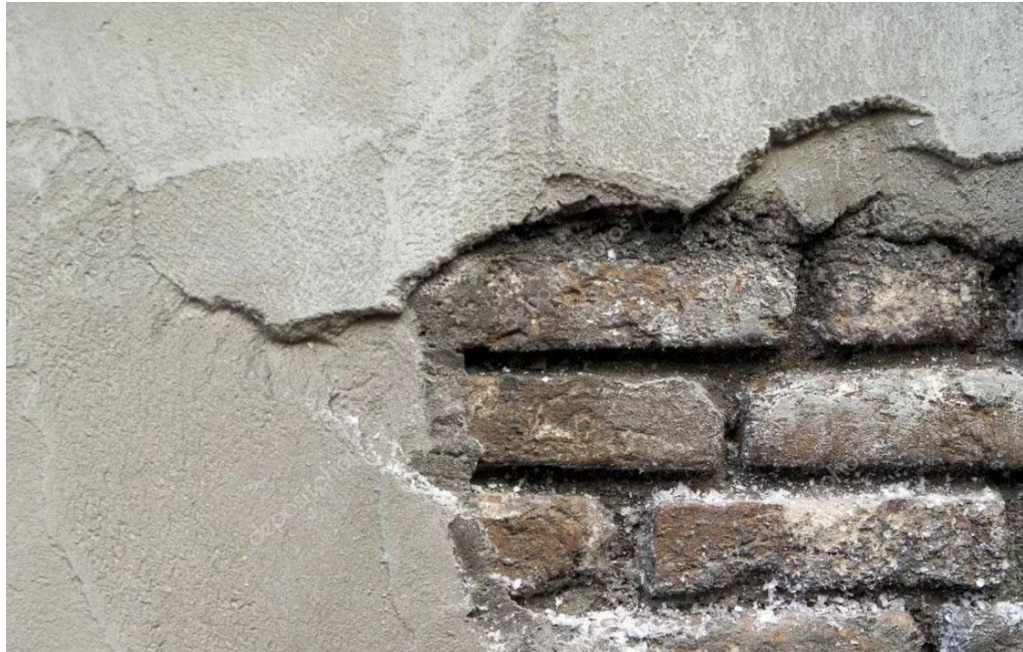
Figure 1. The outer wall is damp from soil moisture.
