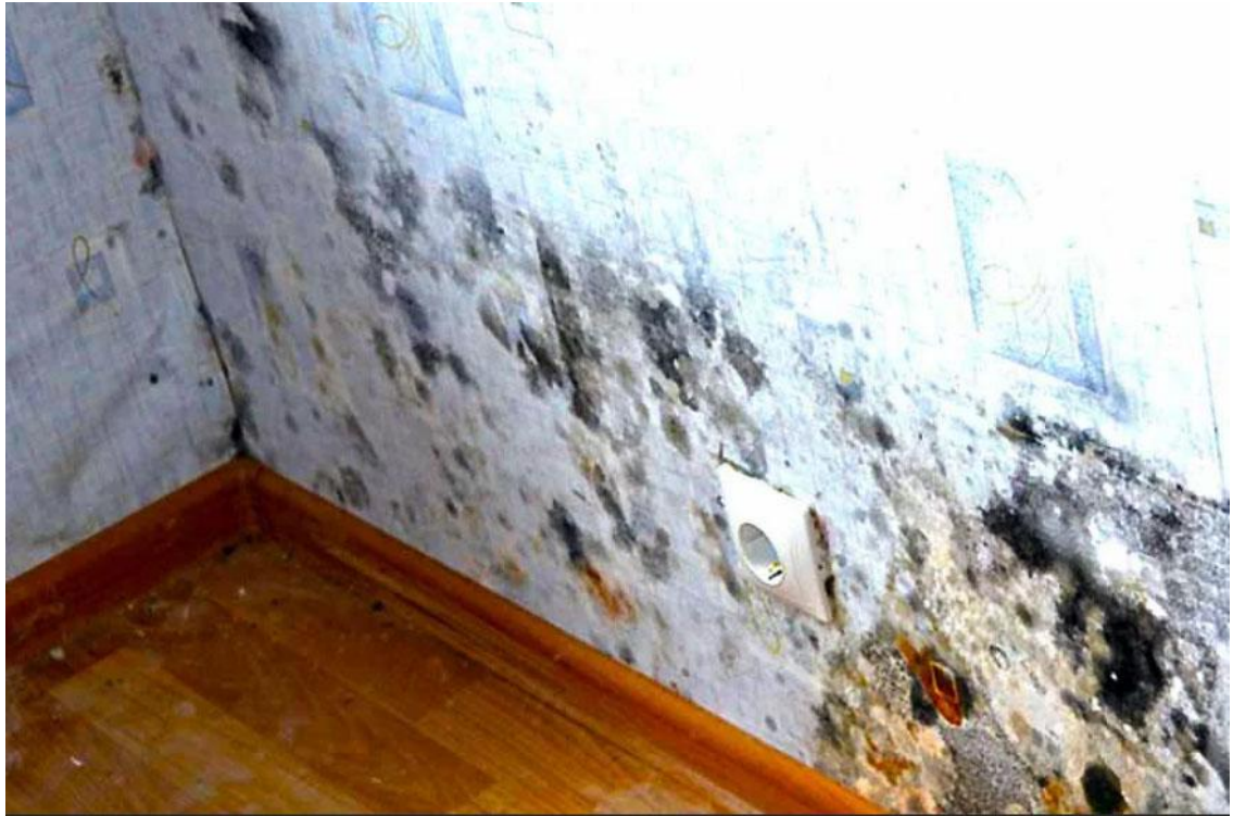
Figure 2. Mold and fungi on the inner surface of the damp outer wall
