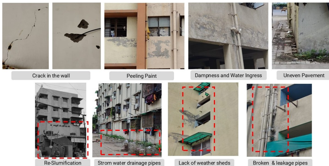
Figure 7. Showing the existing technical inadequacies.
