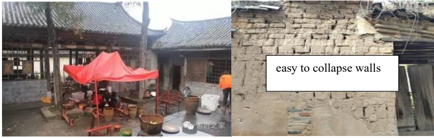
a. Temple activity place b. Easy to collapse walls
