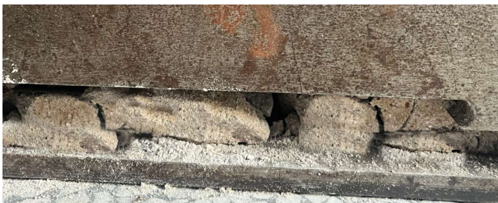
Figure 2. Roof Caving Morphology
