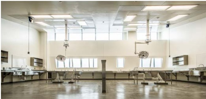
Figure 2. View of two open south facing bays. The autopsy facilities consist of eight open bays, two isolation bays, anthropology laboratory, teaching theatre, and a tissue recovery suite. © 2023 Government of Ontario. Reprinting or reproduction of this material is not authorized.
