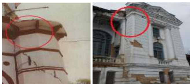
Fig. 4. Separation of facade
