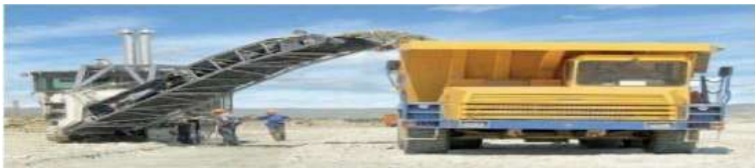
Figure 9 Conveyor loading system
