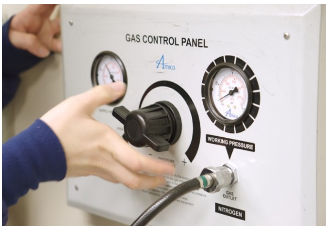
Figure 1. OR wall gas (nitrogen) outlet. (Used with permission from the Children's Orthopaedic Center, Los Angeles)
