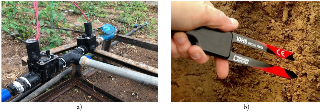
Figure 1. Solenoid valves (a) and soil moisture sensors (b) used for the designed automatic irrigation system
