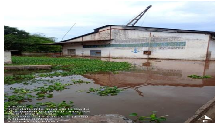
Figure 11: Flooding of ONATRA facilities on the banks of the Kwilu River in Kikwit, November 2023.
