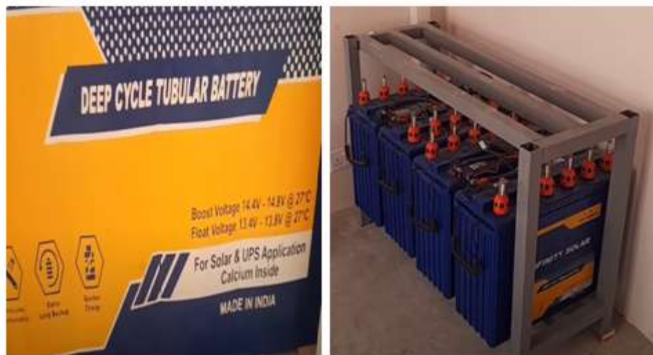
Image 4: The stored electricity battery
