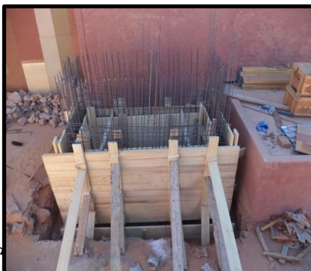
Figure 12: Picture showing the first stage of casting the wall of the water tank.
