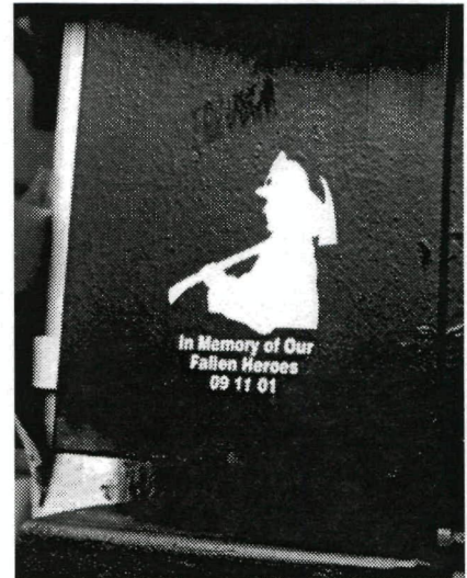
This image was stenciled on an electrical box near Ground Zero
