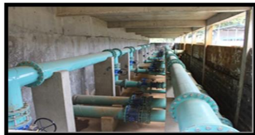
Figure 11: Overhead Water Pipelines
