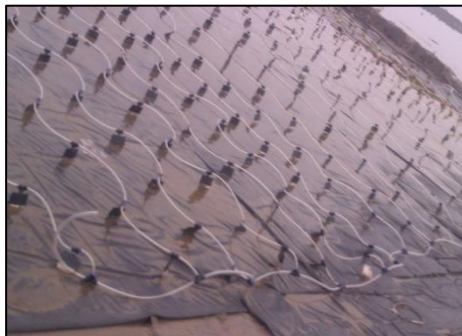
Fig 6. Vacuum gas pipe area
