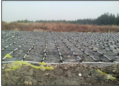
Fig 5. Vacuum filter pipe area
