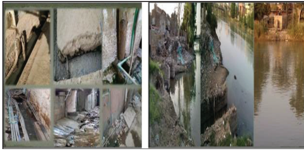
Fig-2: Schools water supply pipes laid parallel with sewerage drains (Right), Excreta discharges into canal & supply pipe (Left)
