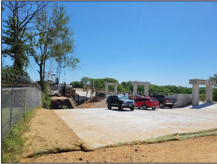
Figure 5. One year into the construction phase, Lake Dunlap Dam. A photo of construction on the Lake Dunlap Dam. May 26th, 2022. Photo by Andrew Adams.
