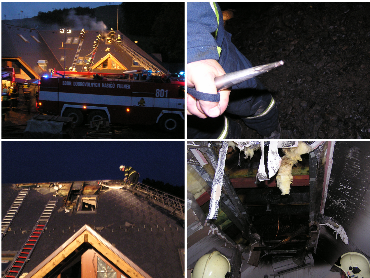
FIGURE 2. Fire at a hotel which was supposedly protected by an ESE conductor.
