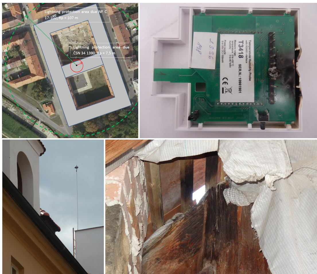
FIGURE 3. Fire at a hotel which was supposedly protected by an ESE conductor.
