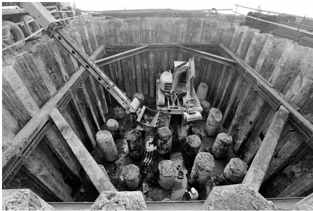
FIGURE 3. Exposed piles in a sheet pile sump
