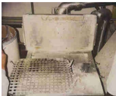
Figure 3: The grid on the chute of the hopper
