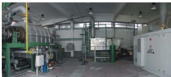
Figure 2: Integrated Pyrolysis Regenerated Plant (IPRP)
