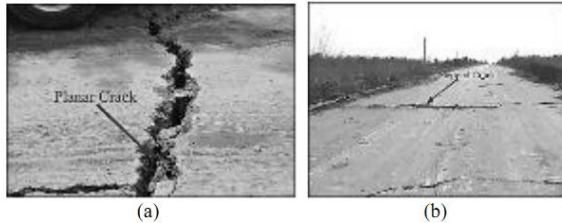
Figure 2: Shape of cracks. (a) Shape of planar crack; (b) Shape of stepped crack.
