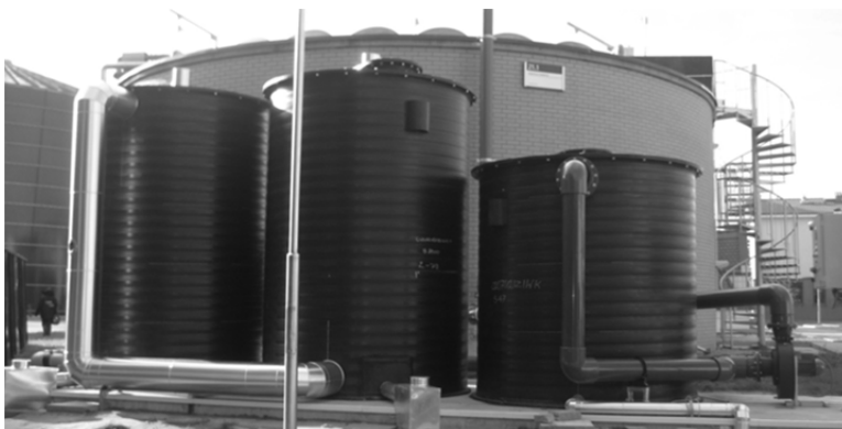
Figure 2: Odour removal installation tested
