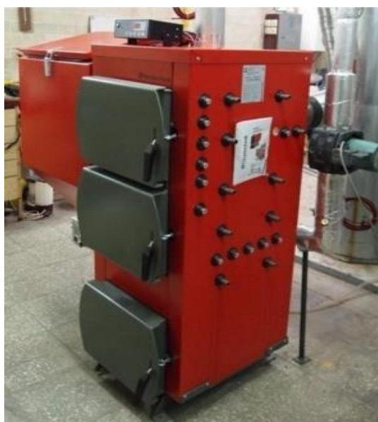
Figure 1: Example of a boiler with automatic fuel supply
