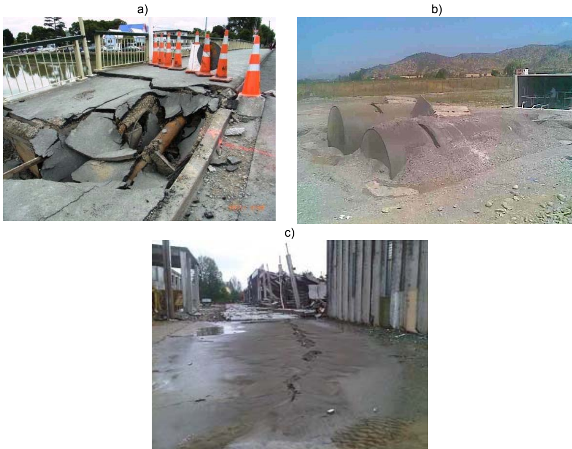
Figure 1: Damage to industrial components induced by liquefaction during recent earthquakes: a) steel buried pipelines in the Christchurch (NZ) earthquake in 2011 (Yamada et al. 2011); b) uplift of a LPG buried tanks during the Chile earthquake of 2010 (GEER, 2010).; c) lateral spread in an industrial district during the Emilia, Italy, earthquake in 2012 (GdL, 2012; GdL AGI, 2013).
