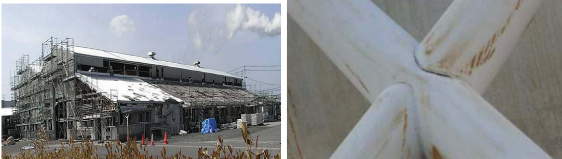
Figure 3 Damage to exterior walls and glass windows from a hydrogen explosion and the steel pipe brace welds of a 2,000 t tank
