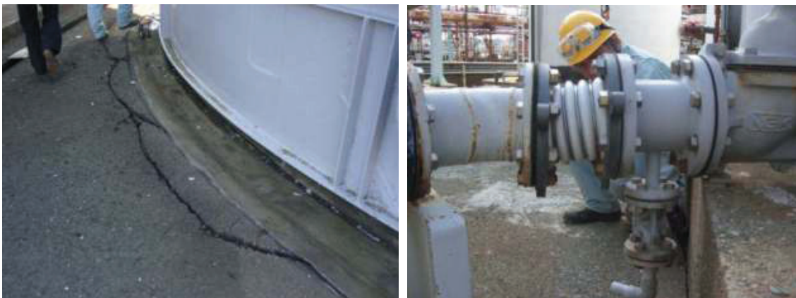
Figure 5 Uneven settlement of the base of a 2,000 kL heavy oil tank and pipe stress due to uneven settlement
