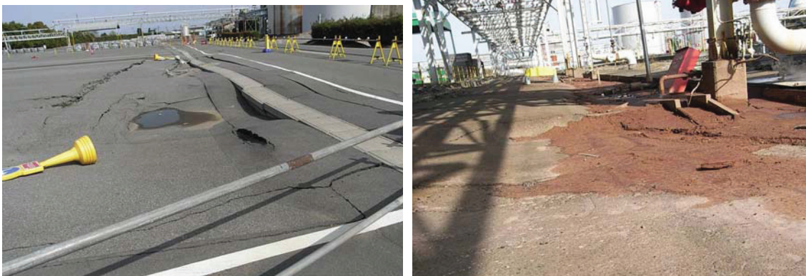
Figure 4 Road caving due to liquefaction and road subsidence below pipe racks due to liquefaction (no damage on the pile foundation pipe racks themselves)
