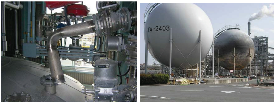
Figure 2 Damage to pipes in the upper section of a container and a hydrogen pipe holder due to pipe damage
