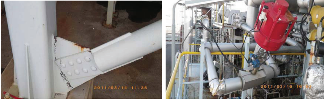
Figure 1 Damage to column base braces and detachment of pipes and automatic valves
