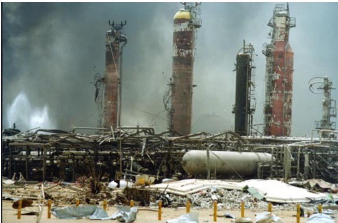
Figure 1 Comparative Blast Damage of Building and Bullet Tank
