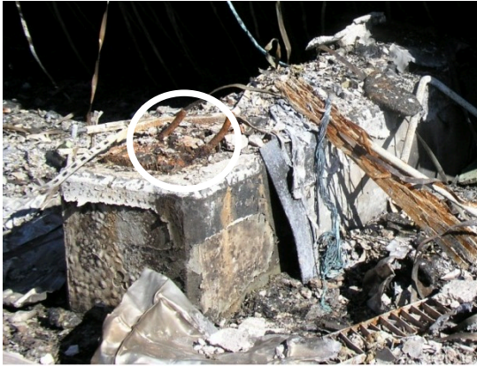
Figure 6 Anchor Failure by Rupture
