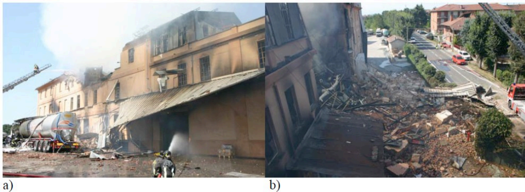
Figure 2 Damage to the main building: a) southern face; b) northern face
