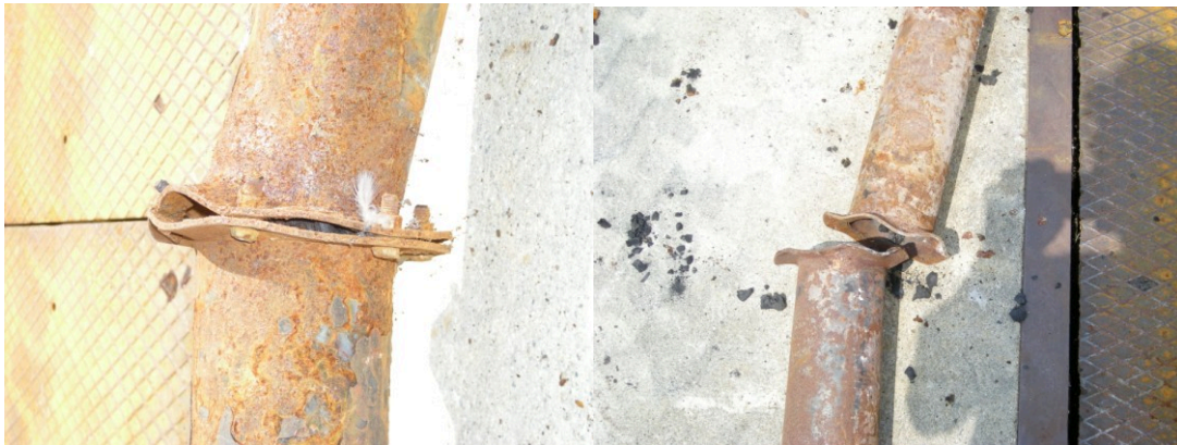
Figure 5 Flanges of the flour discharge pipe
