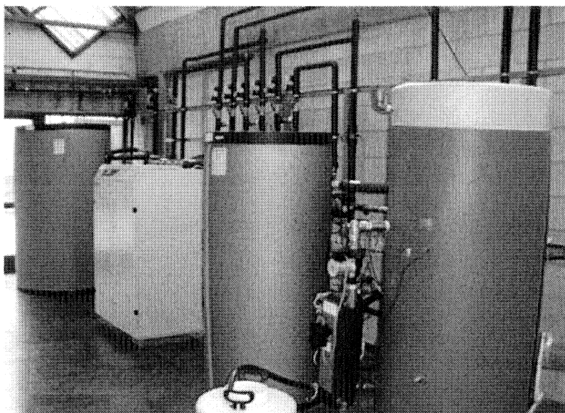
Figure 2: Photograph of the complete installation of heat pump.
