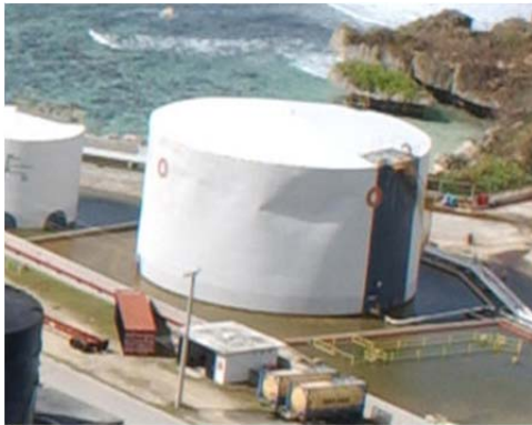
Figure 2: Buckling of a tank in the island of Guam, under a hurricane, 2002 (LEF - Learning from Engineering Failures, s.f.).
