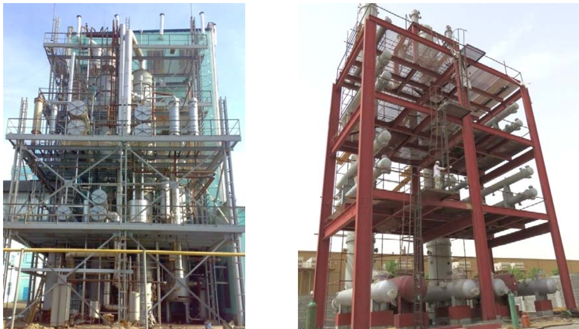
Figure 9: Cyclic distillation column as part of a plant producing ethanol in the food industry (left), and two cyclic distillation dividing-wall columns installed for fractionation of kerosene (right).
