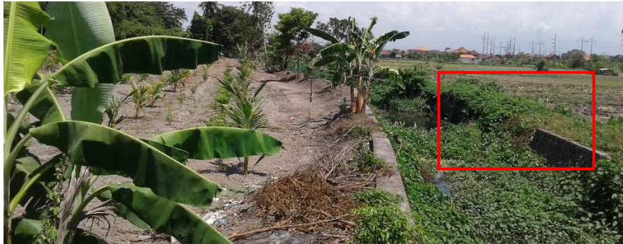
Figure 4. Damage in River Revetment and River Silting
