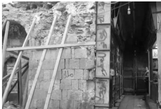
Figure 4. Deterioration of Wikālīṭ al-'Anbariyin's interior. (Source: Dardasha Tareq, 2019. https://www.youtube.com/watch?v=-ZtLLsrwJU8 ) 2015
