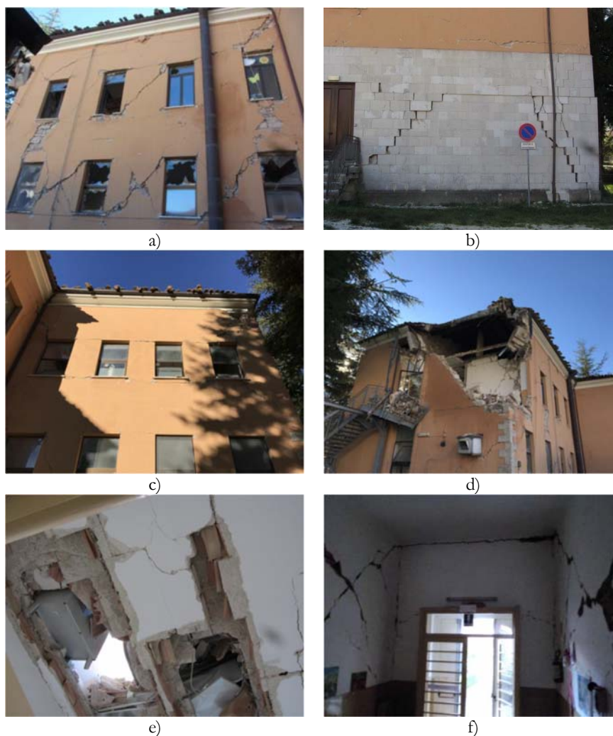
Figure 4: Damage state updated on December 8 th , 2016: a) diagonal shear cracks in piers and spandrels, b) shear-sliding mechanism, c) flexural cracks, d) out-of-plane mechanism, e) local collapse of the slab between the raised ground floor and first floor, f) cracks in correspondence of the connection between walls and slabs [11].
