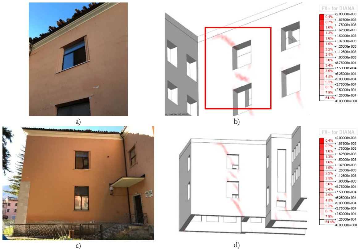
Figure 19: Correlation between the real and numerical damage occurred in the north external walls of body A due to the October 26 th earthquake ( PGA_x = 0.36\text{ g} ): a-b) cracks observed in-situ [11, 12], b-d) crack pattern in terms of principal crack width for a horizontal load of 0.37\text{ g} in -X direction.
