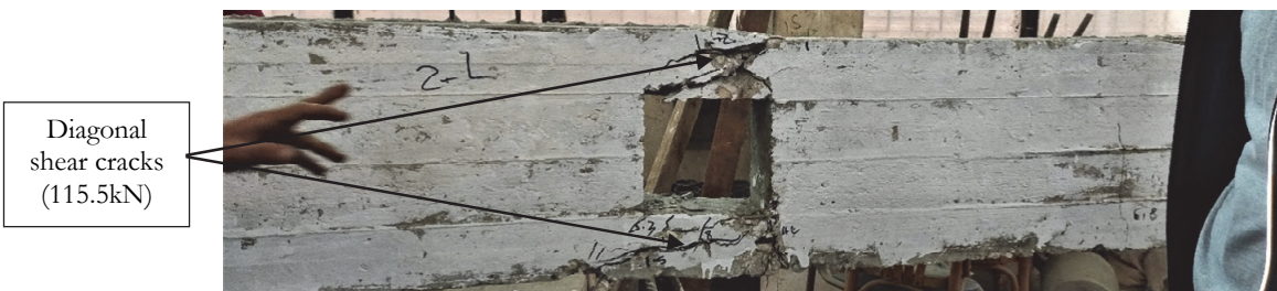
Figure 22: Failure mode for (B2L)
