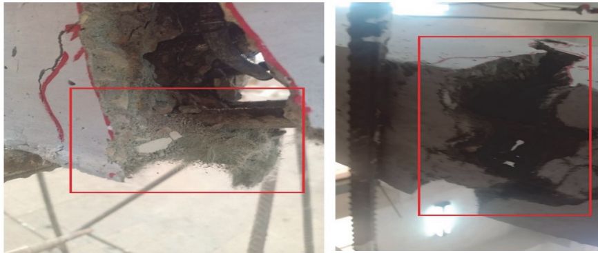
Figure 13: ECC groove rupture at tension surface.
