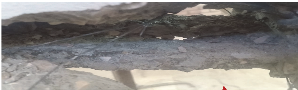
Figure 10: Epoxy groove split from beam.
