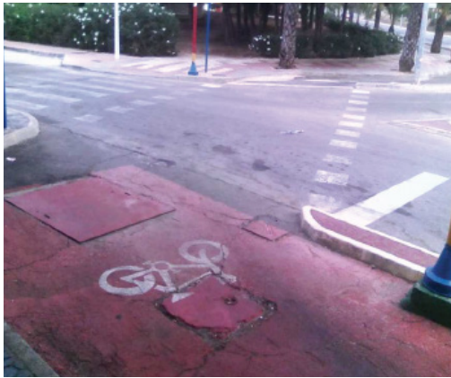
Figure 4. Example of deteriorated bike lane, and lack of maintenance (tourist area)
