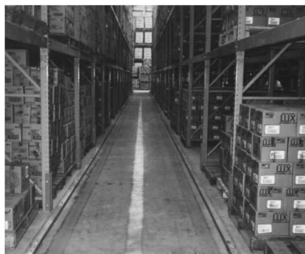
Figure 6. Industrial floor built for rack shelves in a very narrow aisle for swing forklift truck traffic (courtesy of Construdiseños Alta Ingeniería Ltda)
