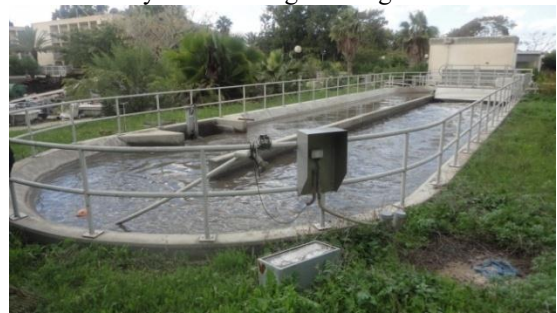
Figure 2: The oxidation ditch under study.
