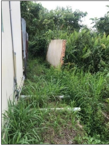
Fig 10. One of the documentation of building damage due to land subsidence
