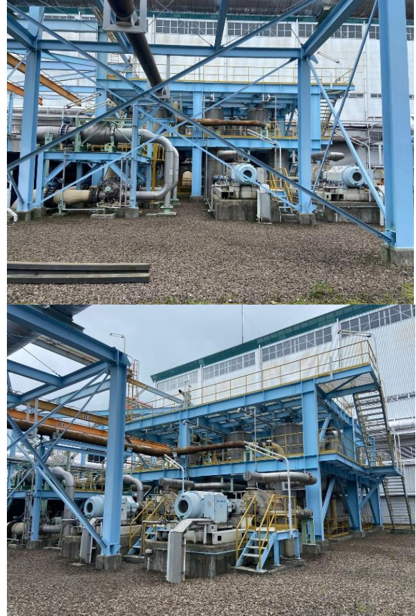
Fig. 2. Gas removal system PLTP Wayang Windu.
