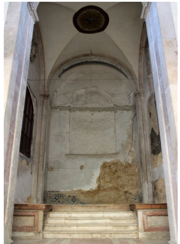
FIGURE 2 | The church's main chapel with 17 th century tiles only on the right wall.
