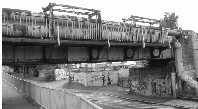
Rys. 4. Widok skrajnego dźwigara, z którego pobrano próbki do badań Fig. 4. The view of the extreme girder from which the samples for testing were used
