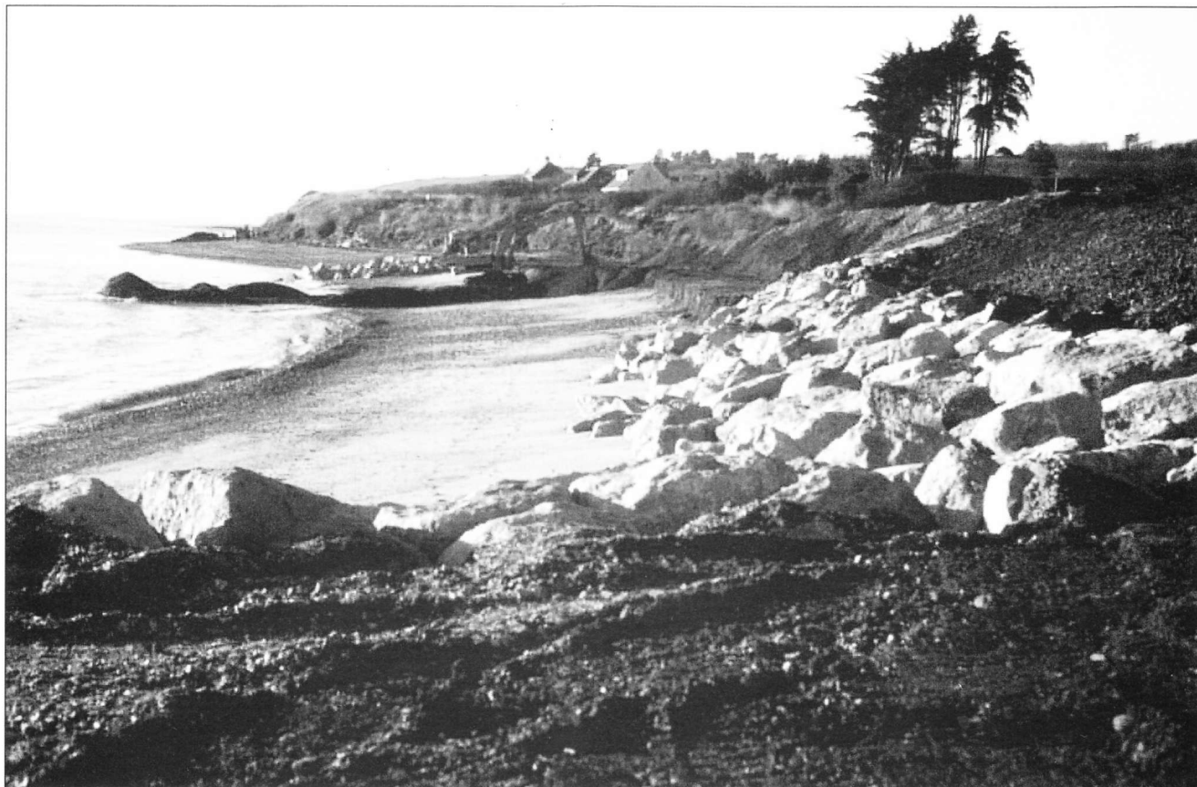
Fig. 1 - The construction of coastal defence structures in progress on a historical stratotype for the base of the Kimmeridgian Stage at Ringstead in Dorset (south west England) – the site is the type locality of the terminal Oxfordian, Evoluta Subzone and the basal Kimmeridgian, Baylei Zone.
