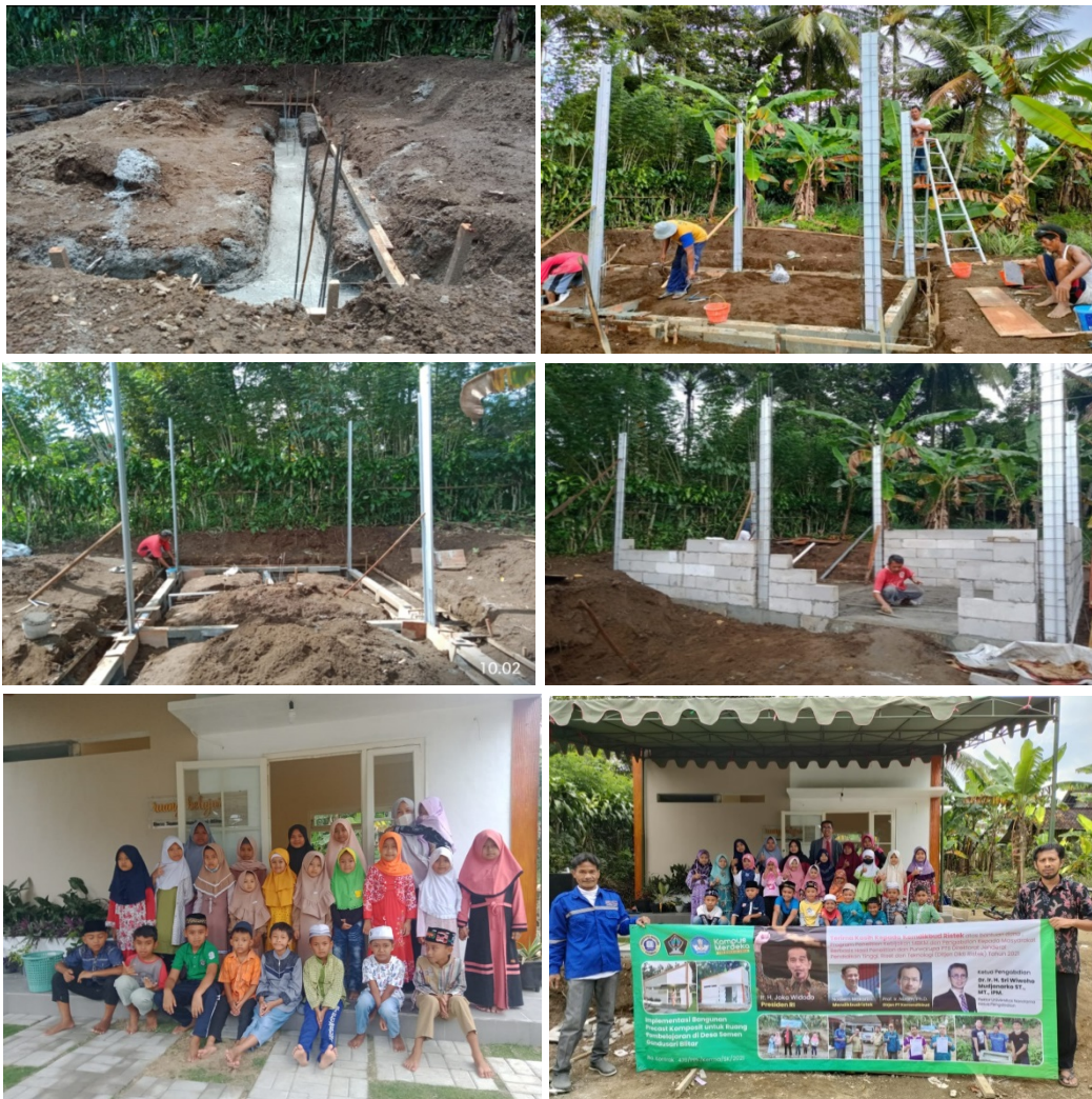
Figure 4. Stages of the learning room construction process along with building drawing designs
