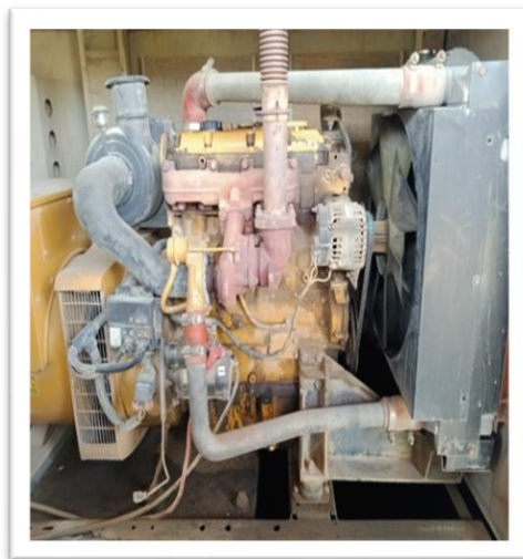
Fig. 6. Inner look of 50KVA AC Generator
