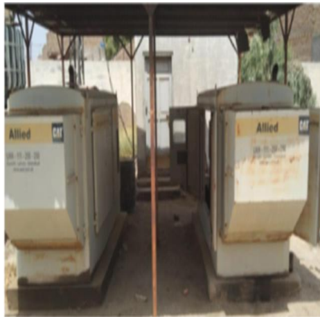
Fig. 5. Parallel Connected Generators at QUEST Campus Larkana
